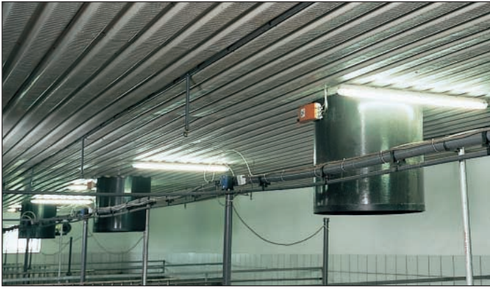
Axial fans in a house with Diff-Air ceiling
