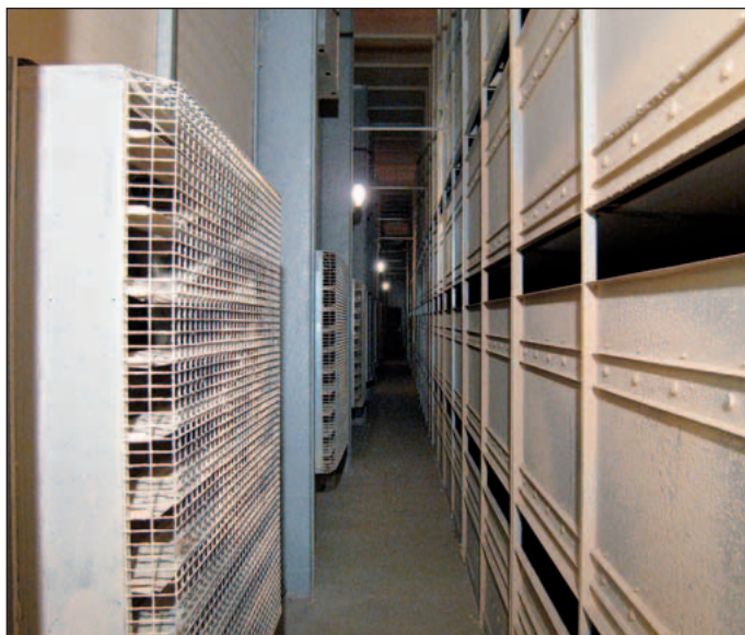
Pressure corridor with an overpressure of approx. 25 Pa
