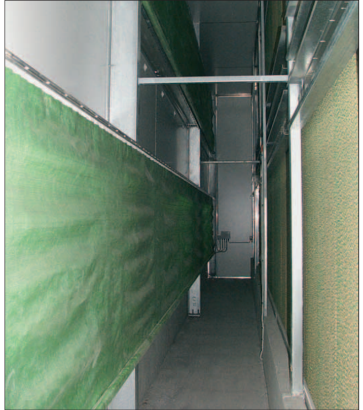
Tunnel inlet with roller curtain
